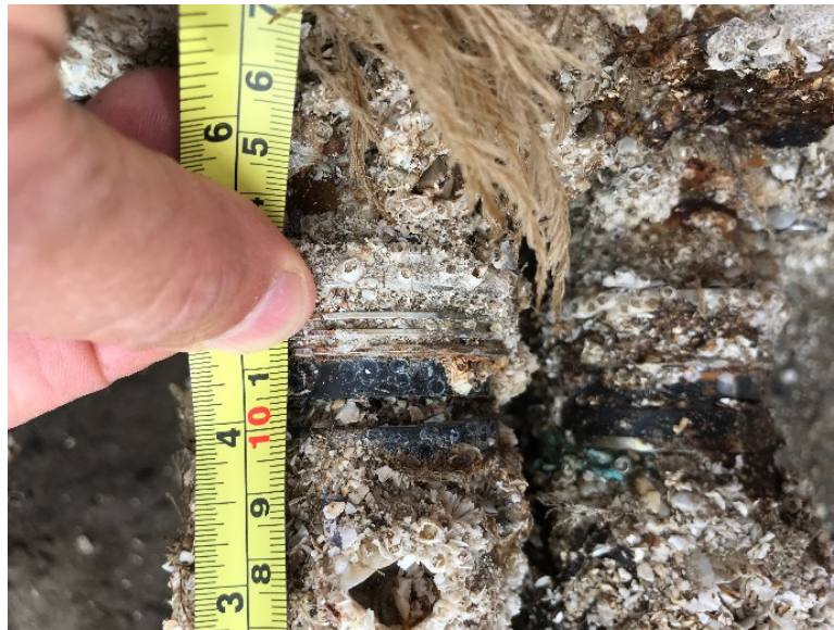
Figure 4. Connectors on the HiCUP junction box. Alloy collars were covering the join between connector ends that are now exposed. These collars have corroded to fragments and the connectors appear to have been pushed apart by barnacles.
